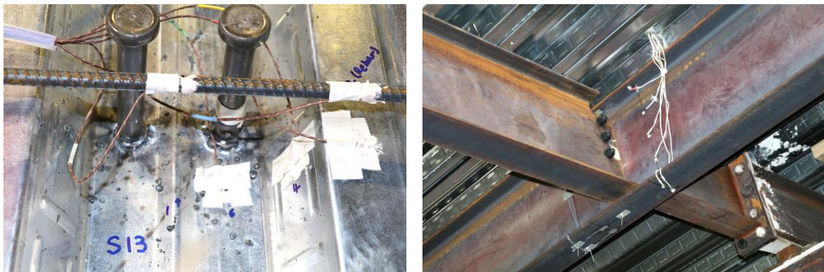
Fig. 53. Photographs of typical thermocouples installed in the composite girder near its midspan.
